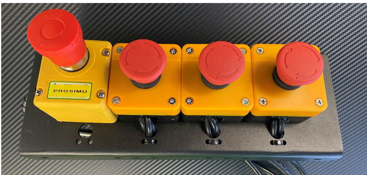
Illustration 50: Emergency stop battery
